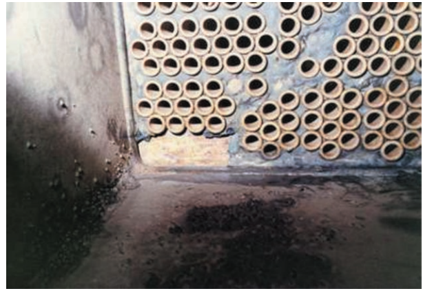
Figure 6. Example coating failure on condenser tubesheet and waterbox.
